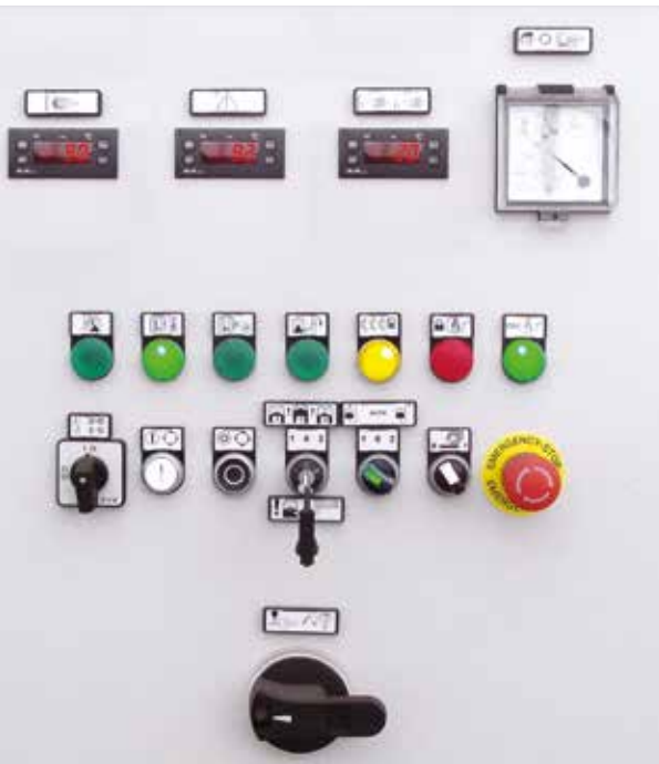
Stationary electrical panel with working devices
