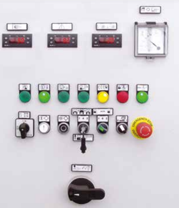
Stationary electrical panel with working devices
